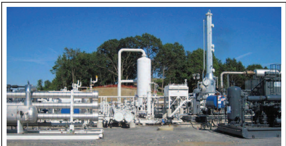
Caiman Energy's new Ft. Beeler 120 MMcf/d cryogenic processing plant was expected to be operational by early December. The company has ordered another 200 MMcf/d processing plant, and expects to order a third plant in the second quarter to expand capacity by another 200 MMcf/d. Located near Cameron, W.V., the facility interconnects with the Texas Eastern Pipeline.
