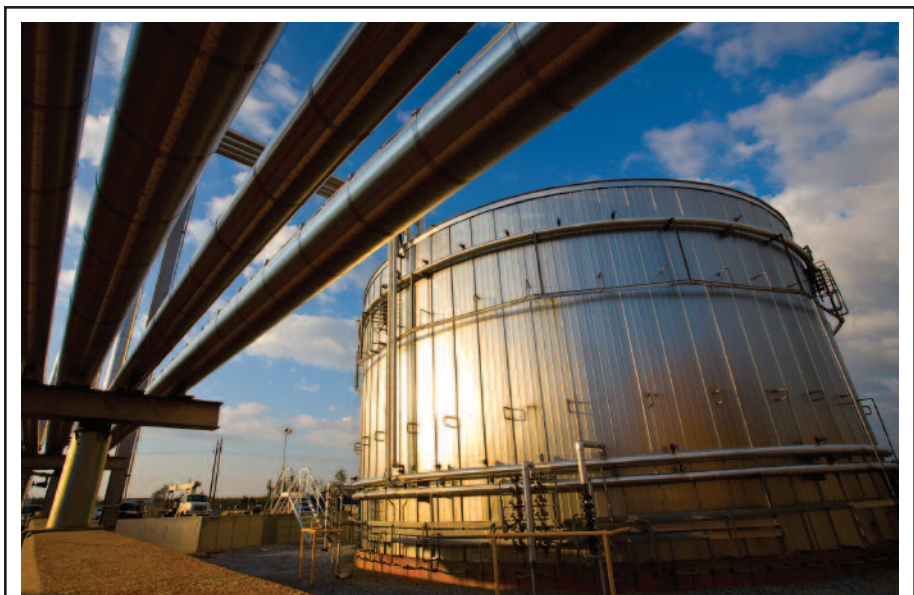
Although it also has upstream operations, two-thirds of Eagle Rock Energy Partners' business is midstream and focused in the Texas Panhandle and East Texas. In the Panhandle, where Eagle Rock has 3,943 miles of pipeline, 137,370 compression horsepower and seven processing plants with a combined capacity of 200 MMcf/d in 10 counties, activity is experiencing a rebirth with horizontal drilling and large multistage fracs in the liquids-rich Granite Wash, Cleveland sands and Tonkawa.
